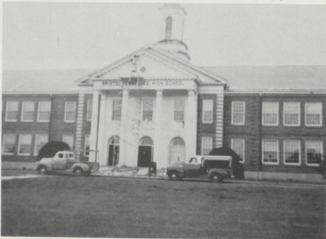
Tennessee High receives a fresh coat of paint by the employees of Cherokee Paint and Wallpaper Company.
